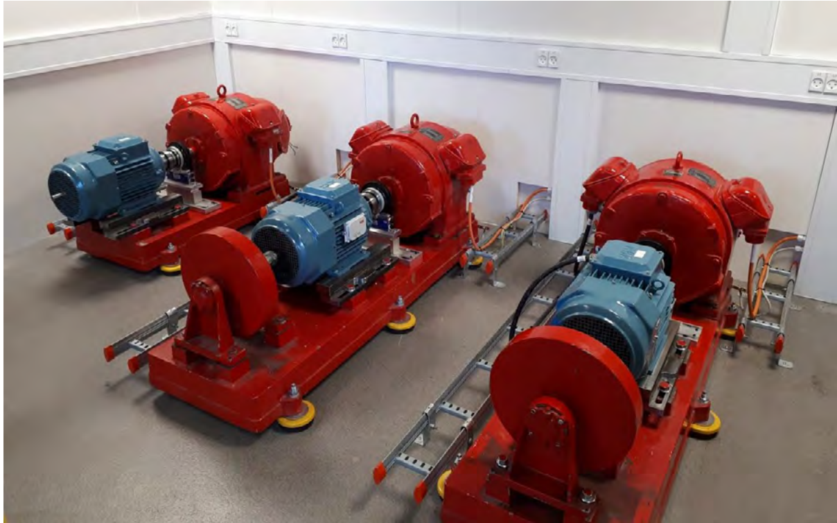
Figure 1 – The three old (red) three-phase synchronous machines connect to three new (blue) three-phase induction machines.
