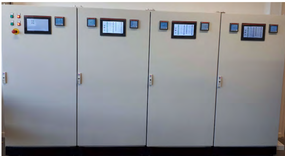
Figure 7 – The four control cabinets +A1...4 for the Microgrid Setup showing the ABB CP600 touch-panel and ABB M2M Digital Analysers.
